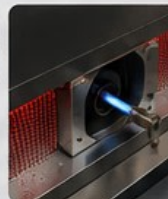
PROPAN GAZ GİRİŞİ PROPANE GAS INPUT
